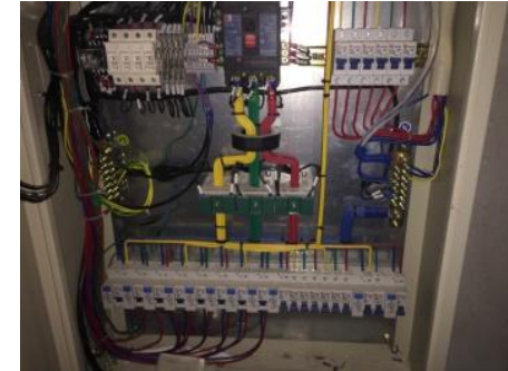
Temperature measurement of terminal distribution box
