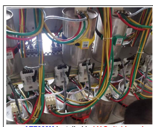
Switchboard Temperature Monitoring Point Showcase
